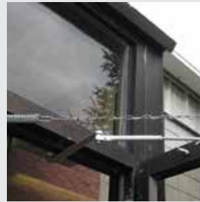
A crash stop was added to this door.
