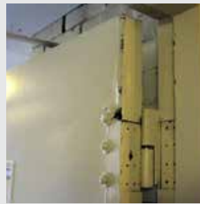
When this hinge failed, it was replaced with a pivot—attached with throughbolts.
