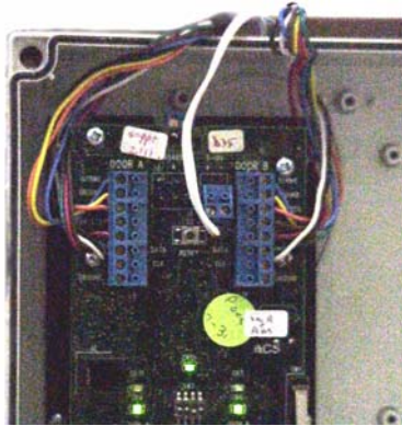
Figure 3-3 – Improper Wire Routing
