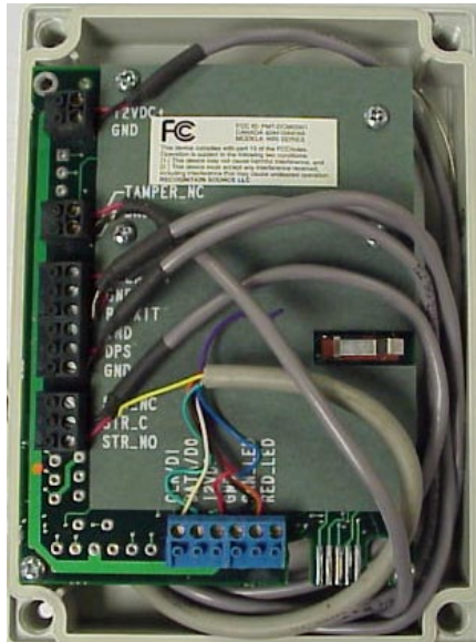
Figure 2-1 – Improper Wire Routing
