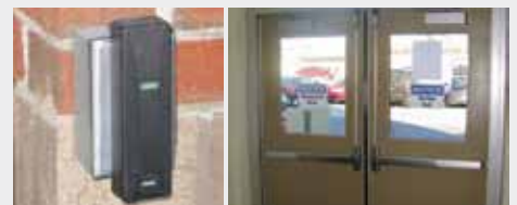
Card reader outside door controls access at selected entrances.
