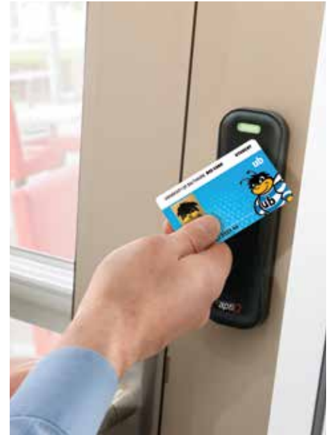
Initially, approximately 70 aptiQ readers were installed on academic and administrative buildings throughout campus.
